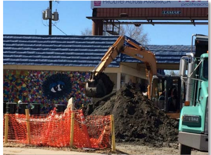
Petroleum impacted soil excavation and disposal is a common Level III remedial activity.
