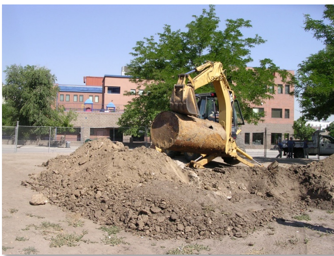
The Level I Site Assessment process begins with removal of a storage tank.
