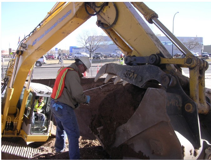
Grab soil sampling from beneath the tanks can be conducted with a backhoe.
