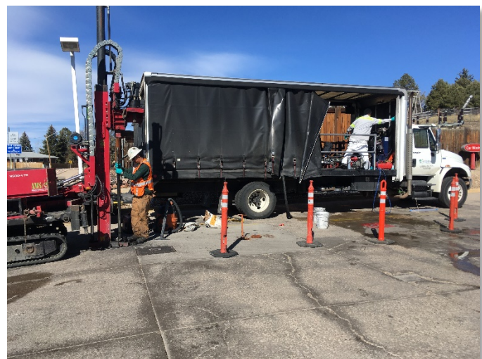
In situ remediation of contamination involves the injection of reagents into the subsurface.
