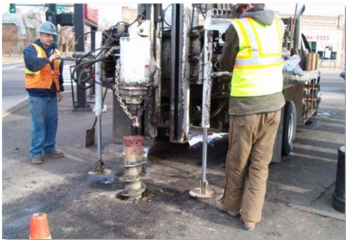
Hollow stem auger drilling is a standard industry practice used to install groundwater monitoring wells.
